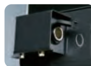
External power outlet
